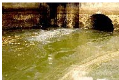
Raw sewage and polluted stormwater impacting Newtown Creek. Credit: (c) Giles Ashford 2005.
