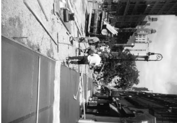
July 1998 Men at work laying new sidewalks and granite curbs on W. 72 St. See p.2.
