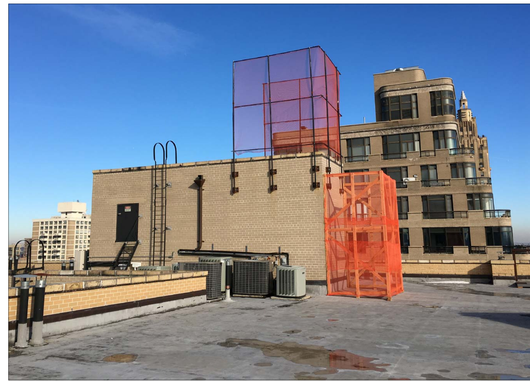
J VIEW OF ELEVATOR BULKHEAD EXTENSION AND NEW VESTIBULE AT THE ROOF
