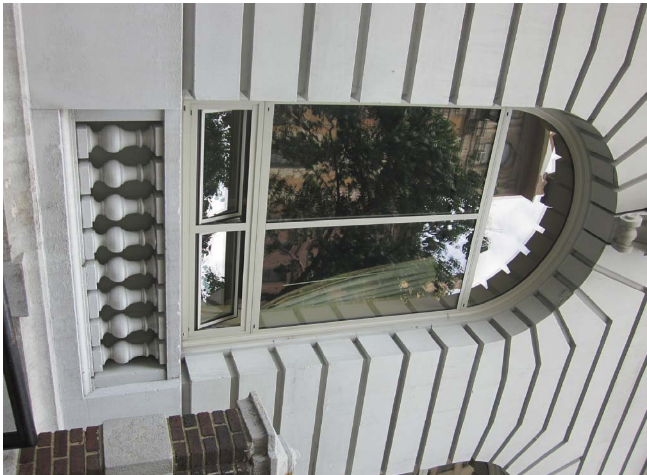
INSTALLED WINDOWS TYPE 1B IN - SWINGING HOPPER FIXED GLASS ABOVE
