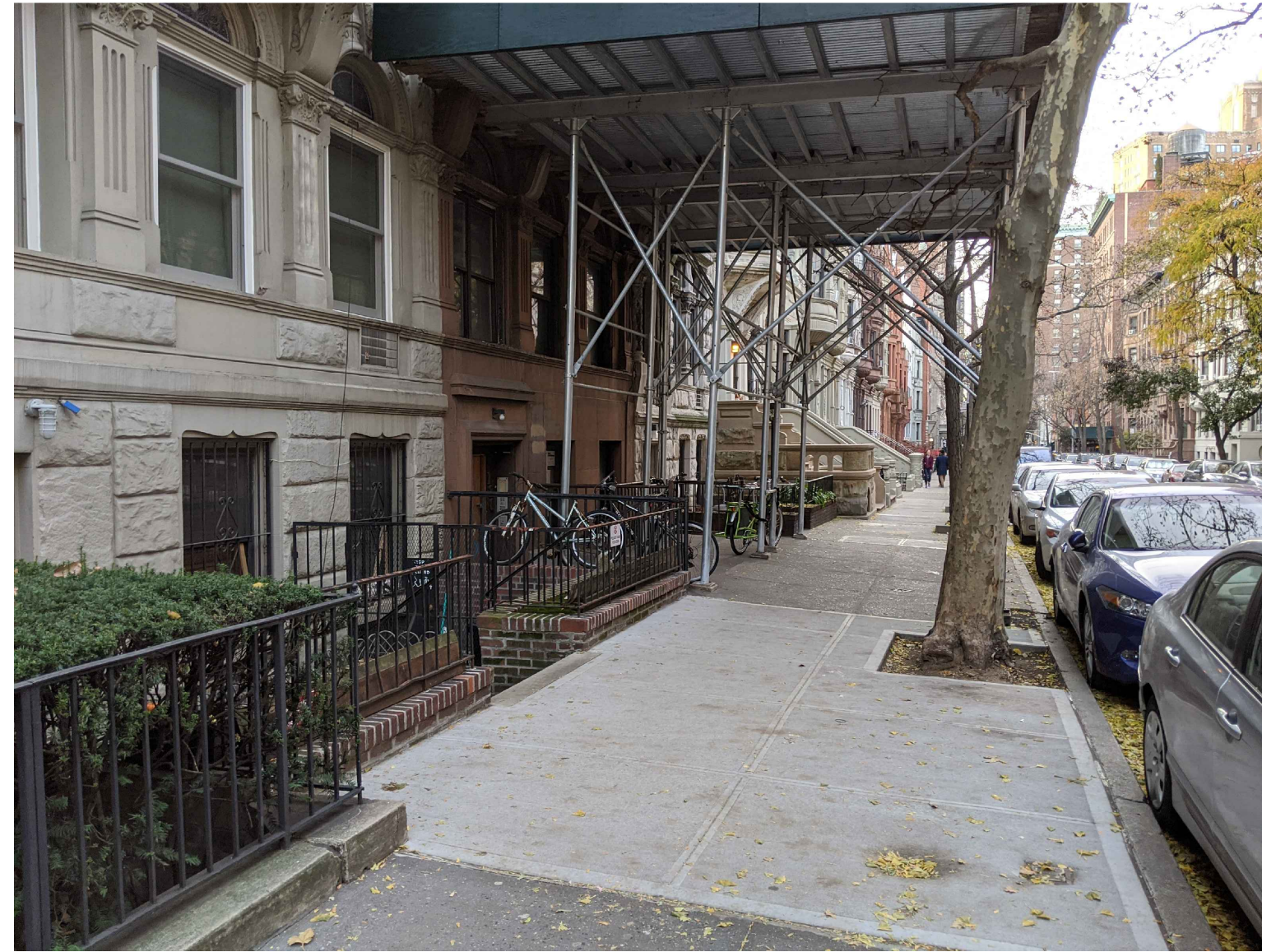
PHOTO @ 118 W 74TH STREET
