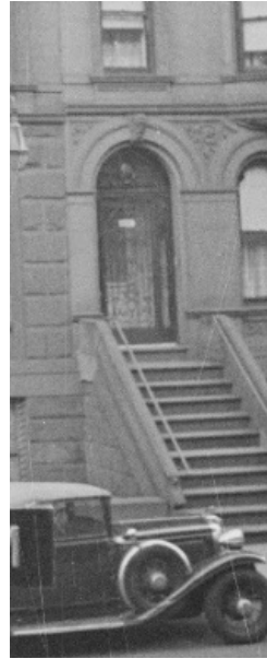
Original 1940 tax photo showing metal and glass single leaf entry door on 309 West 90 th Street
