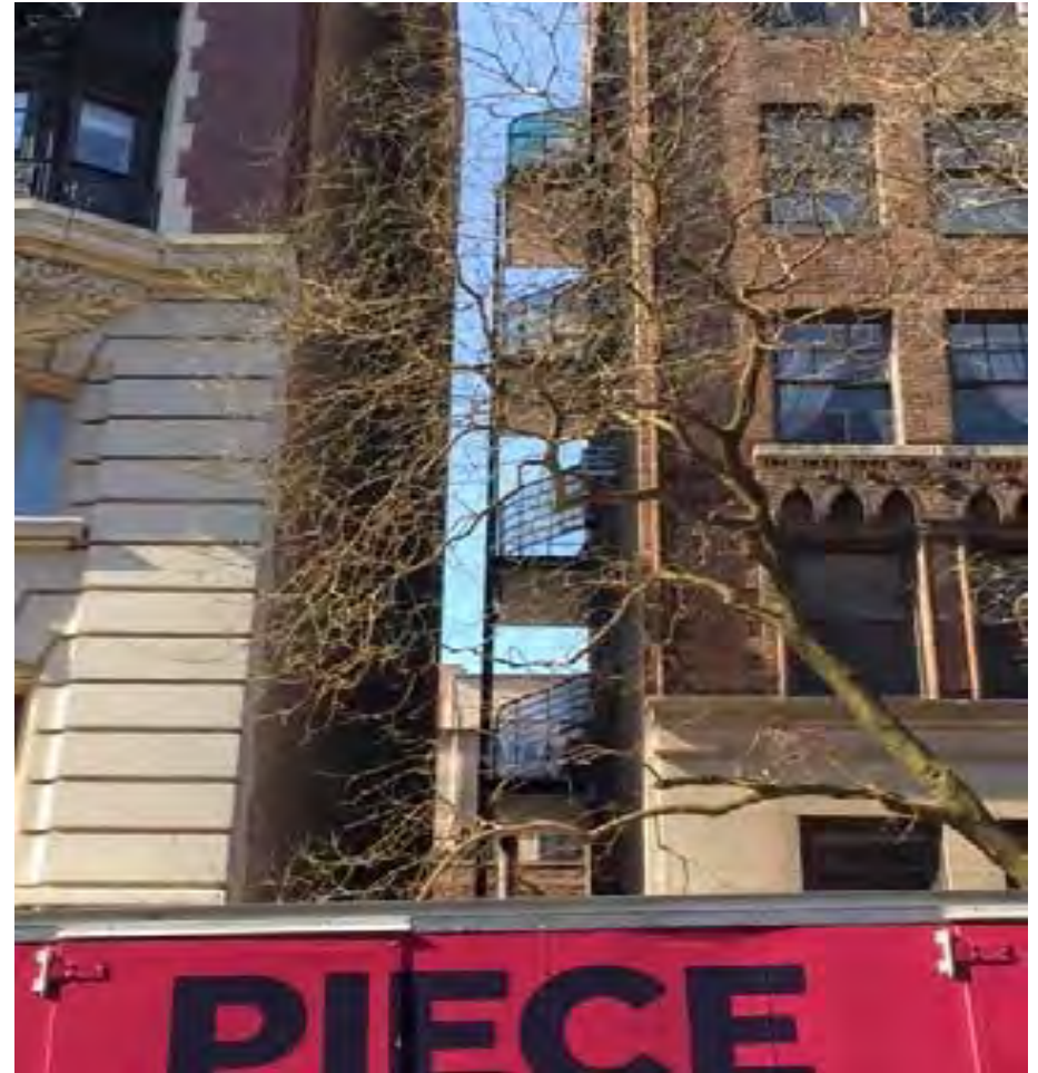
The existing balconies are to be replaced on the 5 th , 7 th , 9 th and 11 th floors.
