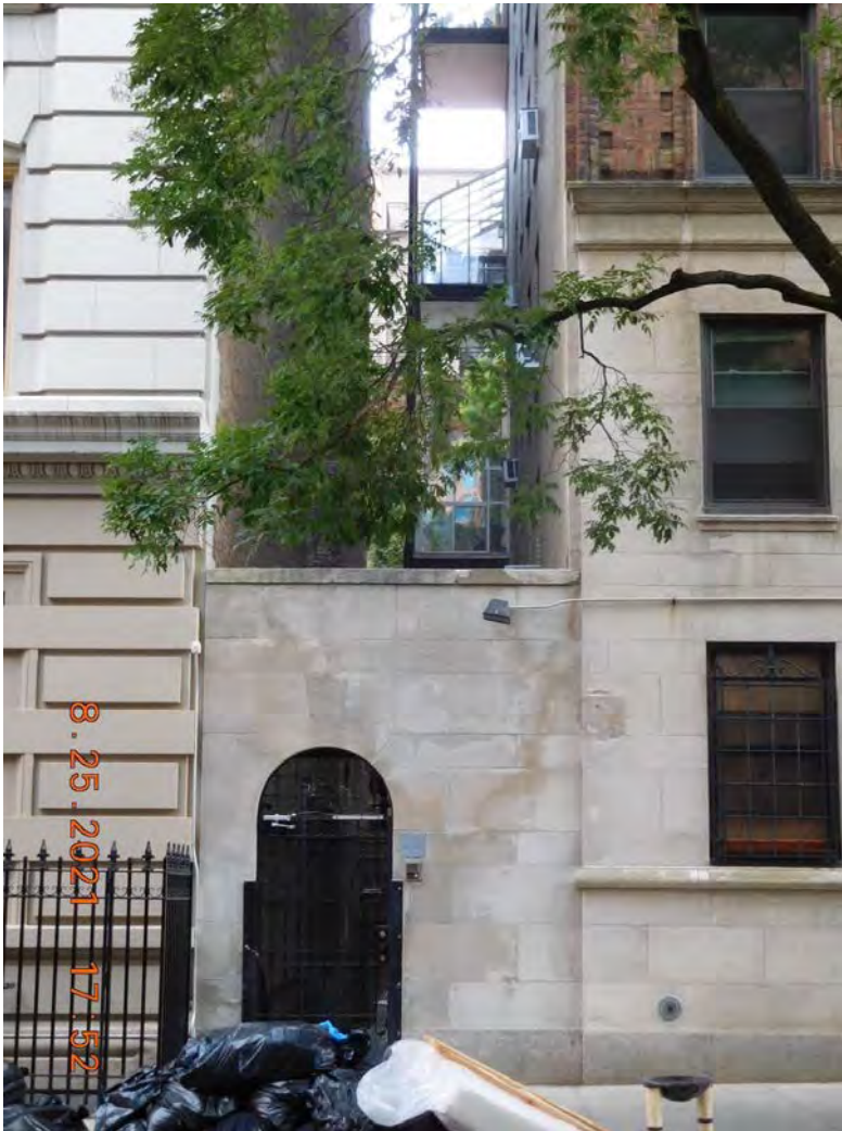
The existing balconies are behind a one story masonry arch and are mid'-block. This photo is taken facing south on West 76 th Street
