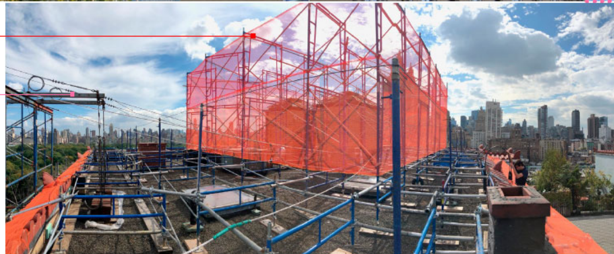
Facade Maintenance Rigging
