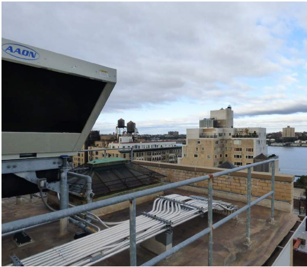
(J) EXISTING EQUIPMENT AND WEST VIEW
