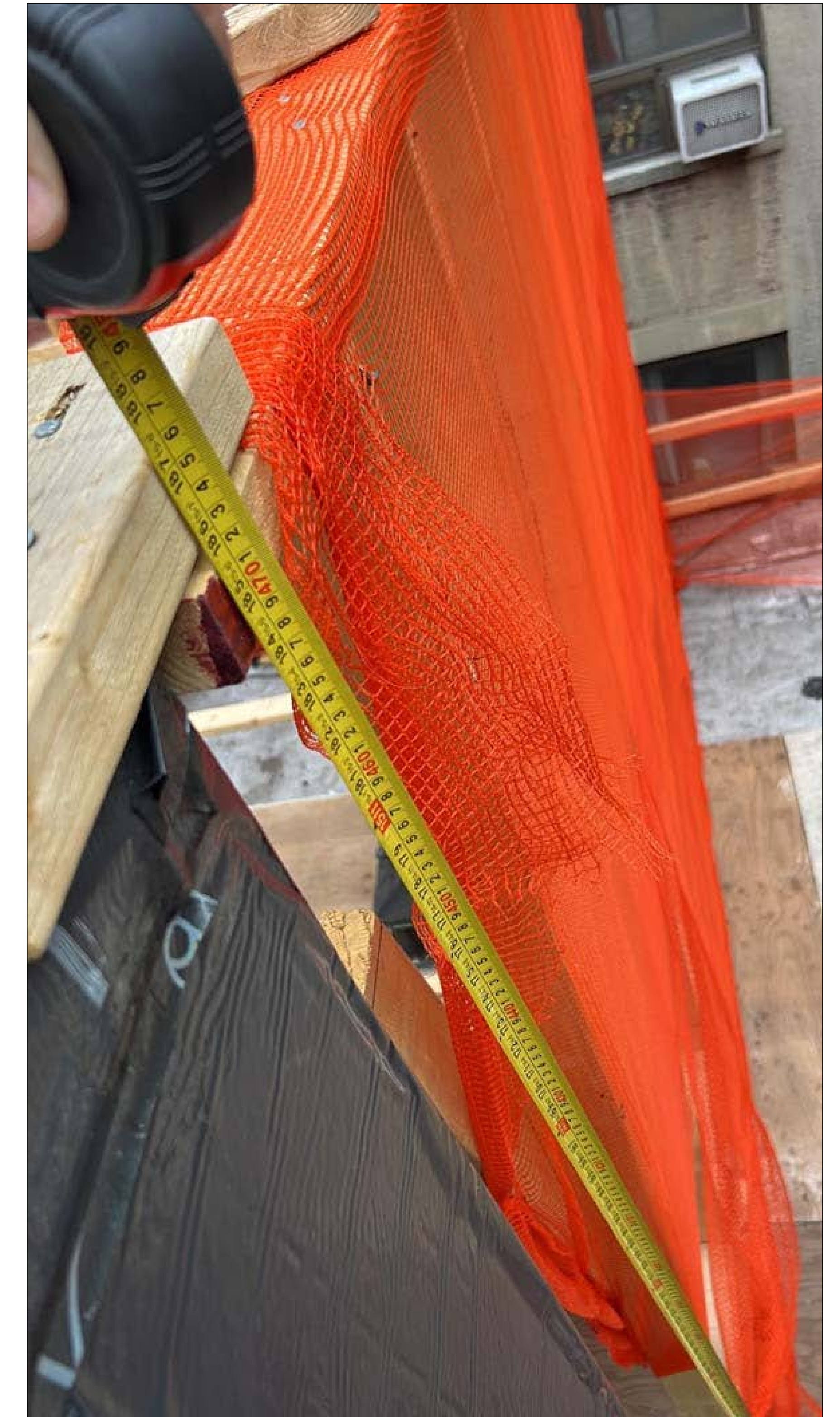
TOP OF RAILING MOCK UP THE MOCK UP CURRENTLY CONSTRUCTED INCLUDES THE HEIGHT OF THE MECHANICAL UNITS. TOP OF RAILING MOCK UP @ 15'-7" ABOVE ROOF AS SHOWN ABOVE
