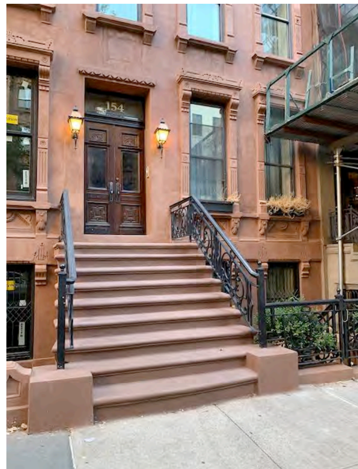
4 CURRENT PHOTO OF EXISTING STOOP 154 WEST 73RD ST. LOOKING SOUTH Scale: NTS
