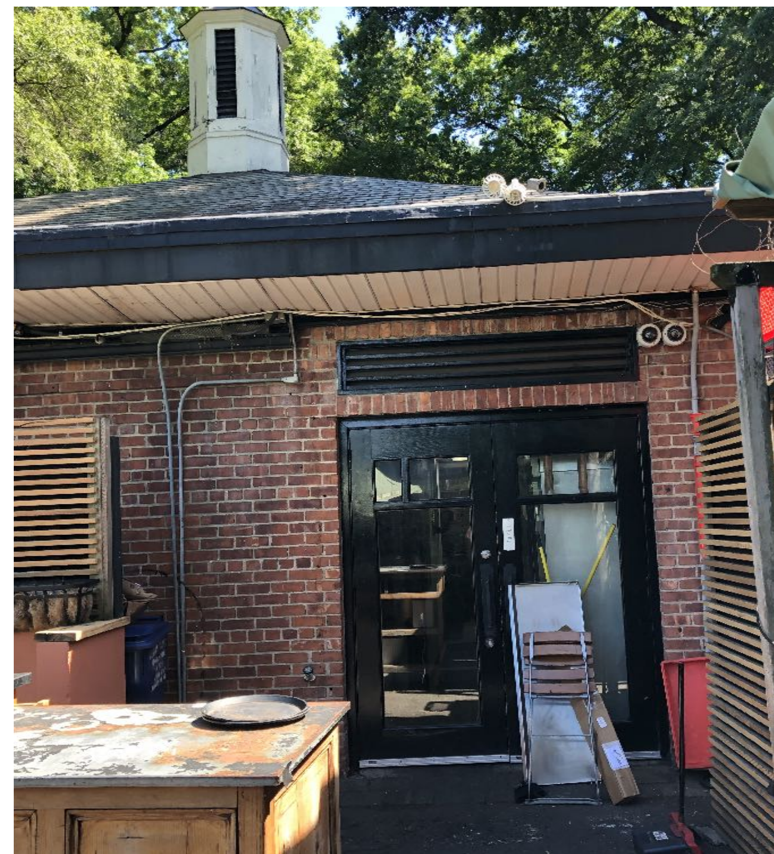
E EXISTING CONDITIONS PHOTO SERVICE ENTRANCE
