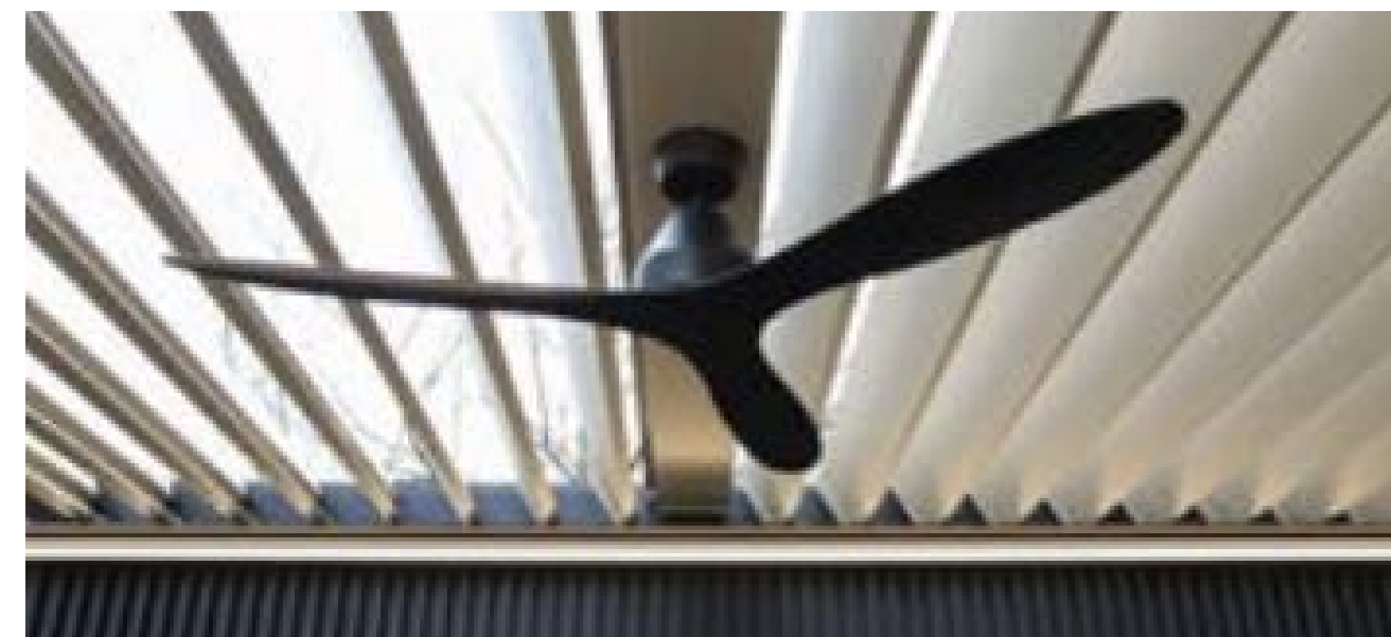
D CEILING FAN MOUNTED TO PERGOLA BEAM
