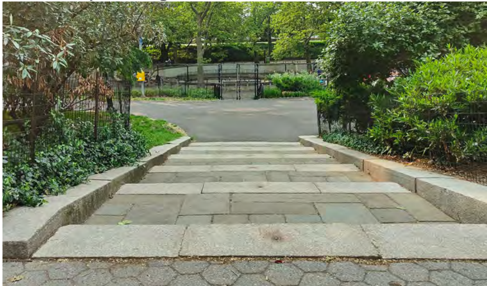
Replace Granite Curb, Bluestone Paver Landings and Granite Stair Treads at Riverside Dr Entry
