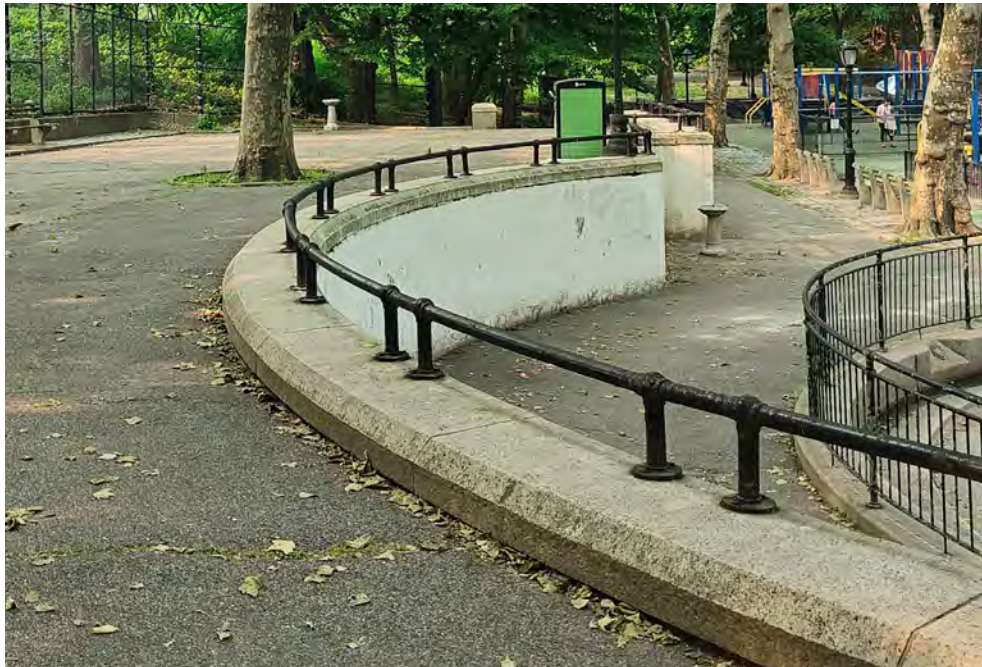
Raise Existing 12" ht Pipe Railing on Existing 12" ht Parapet wall to compliant height
