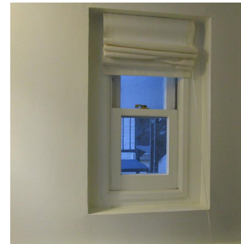
Existing Window Condition - Interior View ㉖
