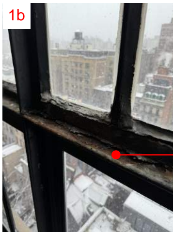
Rust through historic steel
