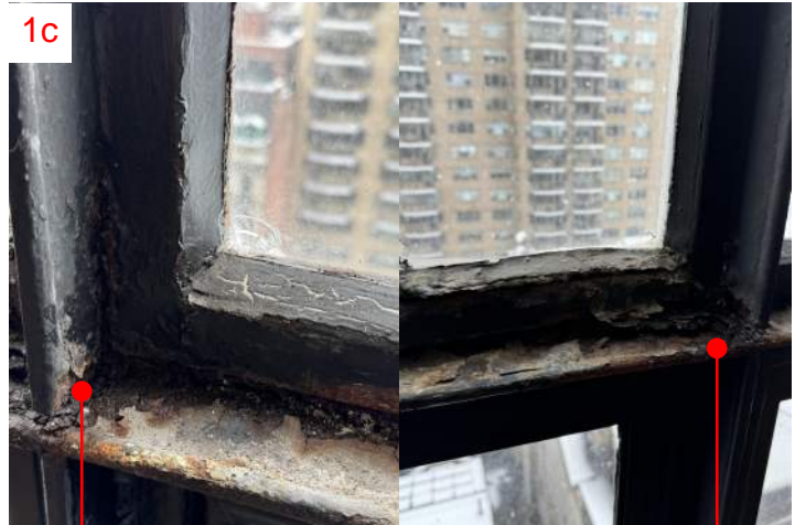
Rust through historic steel structural members
