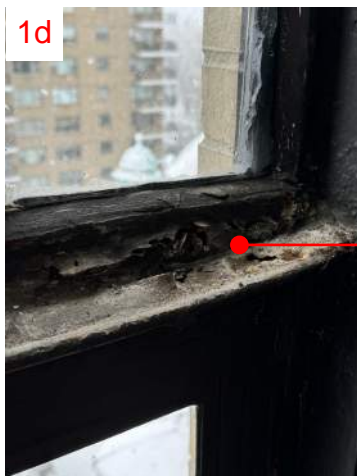
Rust through historic steel
