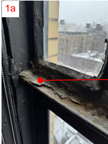
Rust through historic steel
