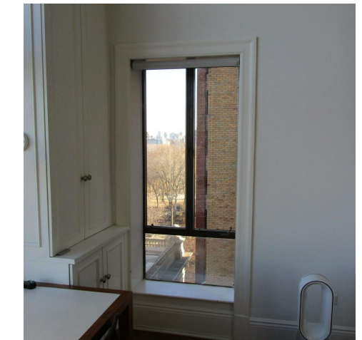
Existing Window Condition - Interior View ㉘
