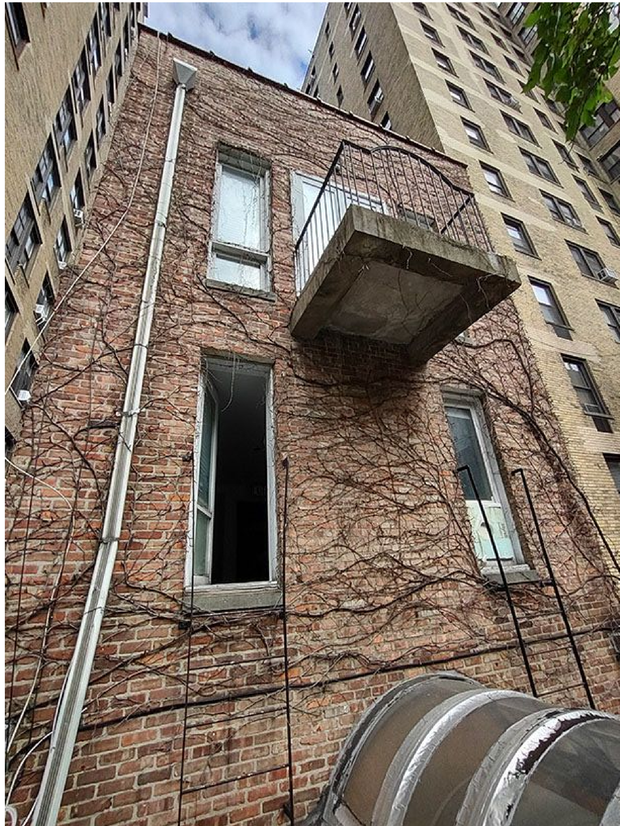
REAR FACADE EXISTING CONDITIONS
